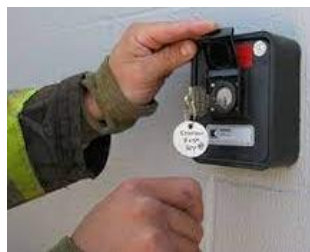
In Some Jurisdictions (e.g. Mississauga) Fire 'Knox' Key Boxes Have Been Approved
